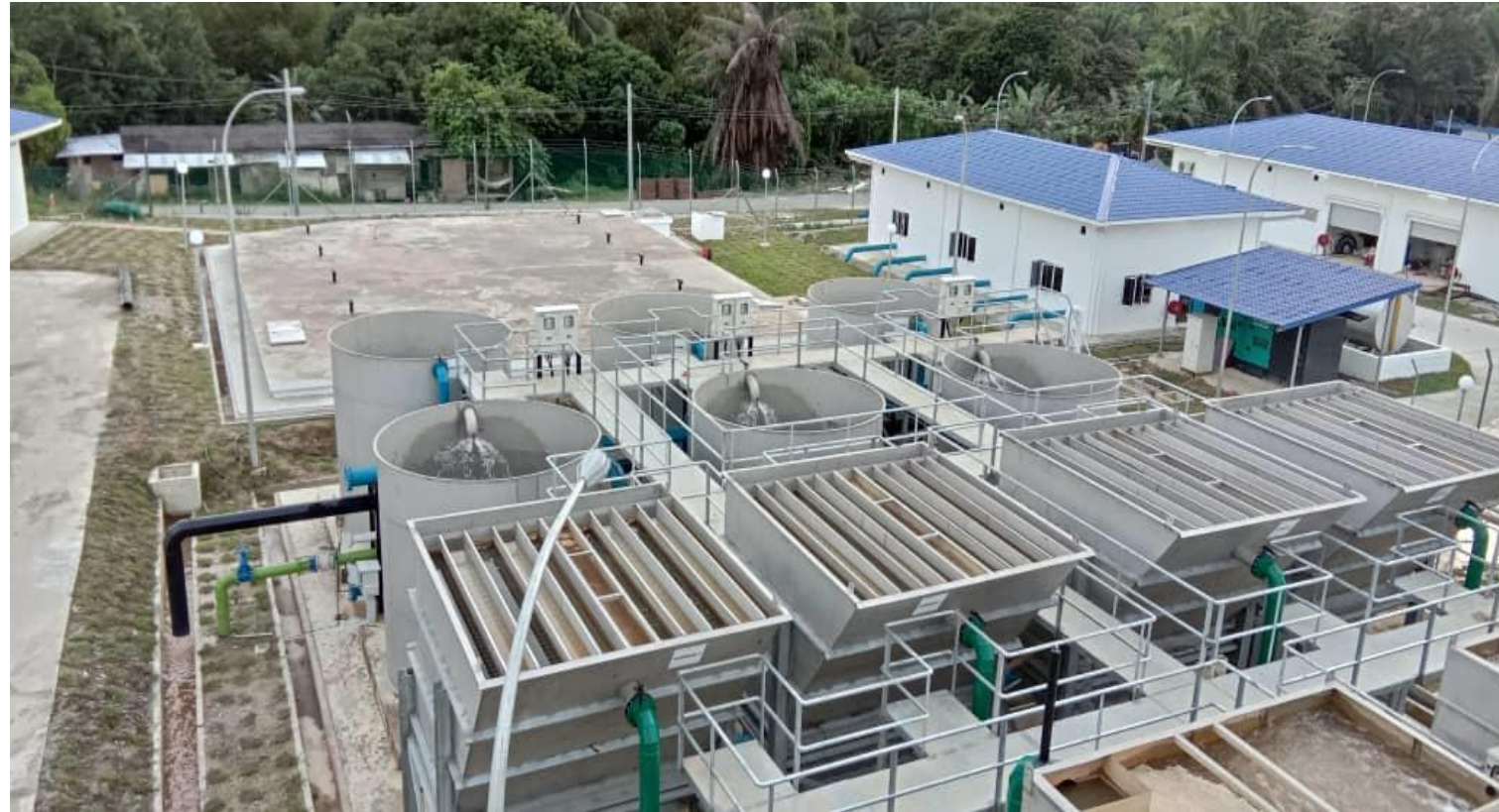
Loji Rawatan Air (LRA) Package Plant
